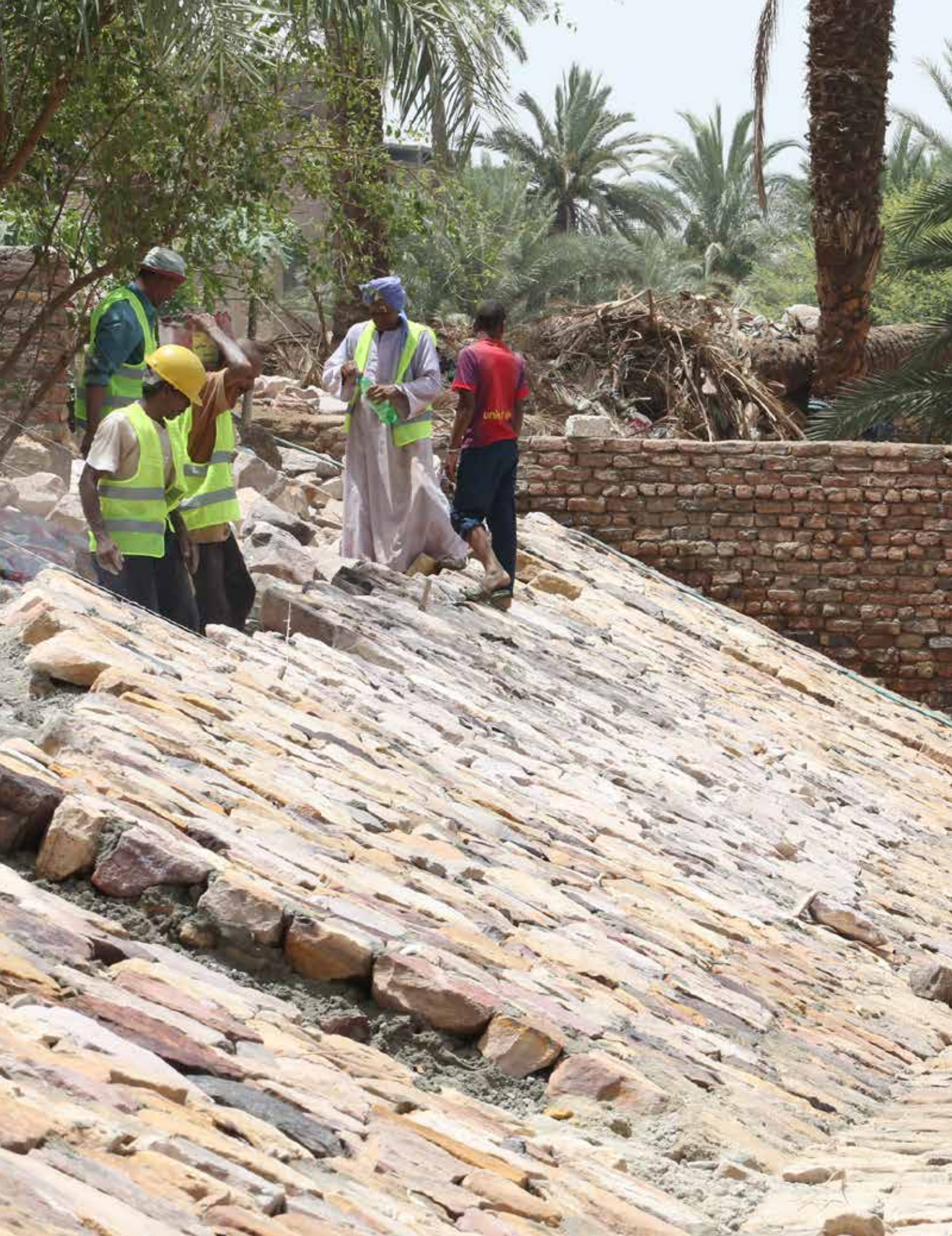
Construction workers in Luxor, Egypt, build stronger river banks along the Nile River. Photo credit: Dominic Chavez/World Bank.
